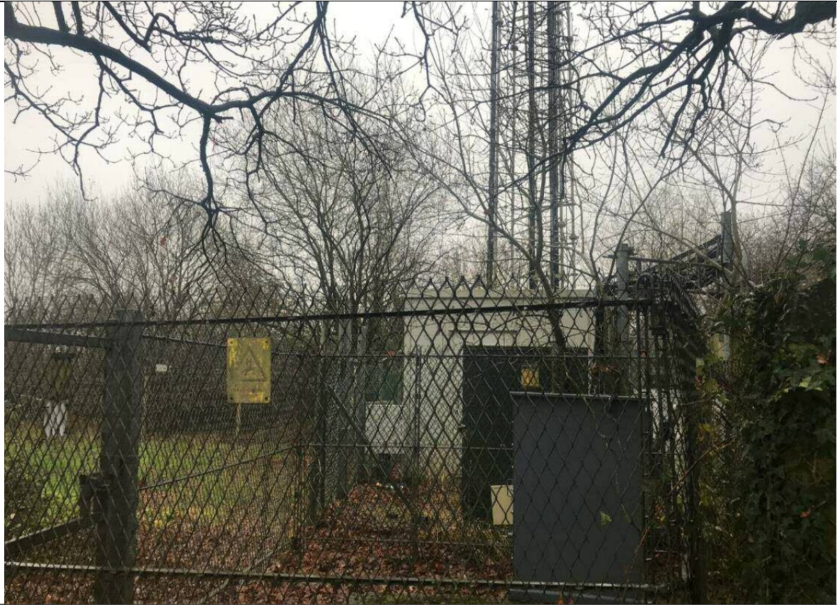
Photo 7: Small electric sub-station against the south site boundary
